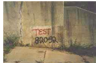
AREA WITH 2 COATS OF LIFETIME™ PLUS AND GRAFFITI WAS APPLIED TO SAMPLE
